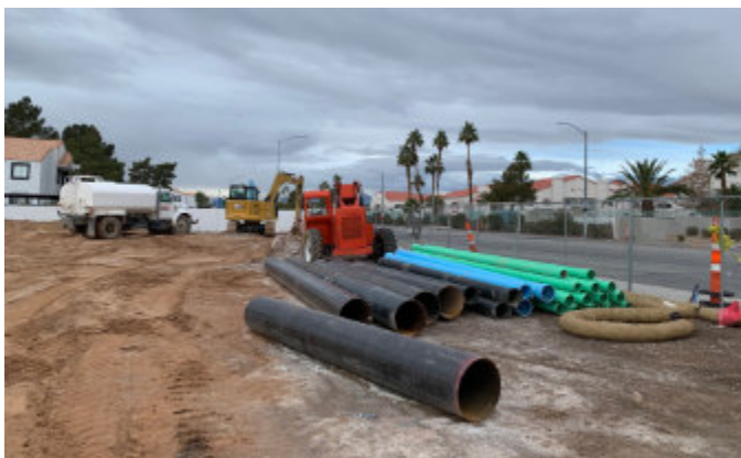
Site preparation photos for construction of Vista Del Sol Apartments in Las Vegas, Nevada
